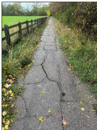
Public Footpath 39/31 Condition
