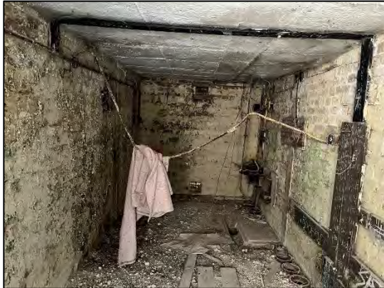
Photograph 1: Example of one of the buildings that displays low potential for roosting bats.
